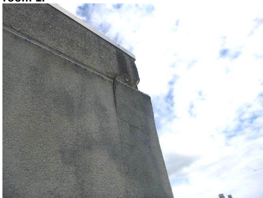
9. Part of the rendered wall coming away from the wall of tank room 1.
