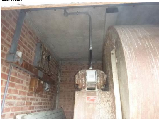
17. Internal view of tank room 2 with a lift room and old water tank covered with pigeon droppings.
