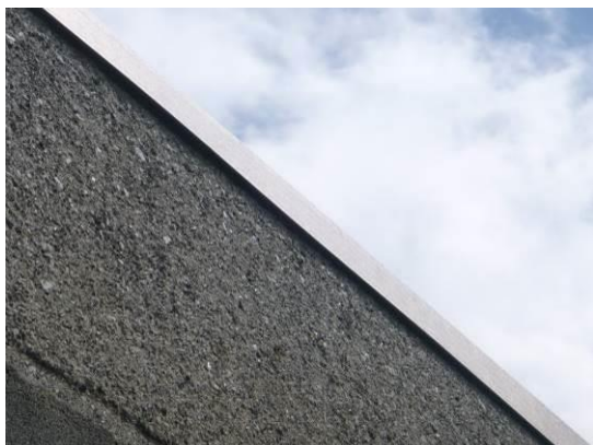
7. Gaps behind some of the fascia's on tank room 1.
