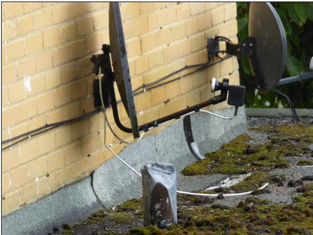
Figure 10. Felt between property and garage roof. 9 Broomfield Road, Tilehurst. 24.09.19
