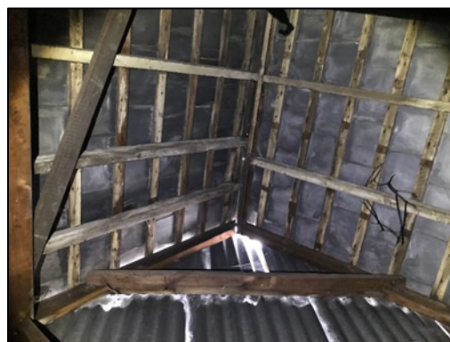
Figure 4 – underside of slates and corrugated tin
