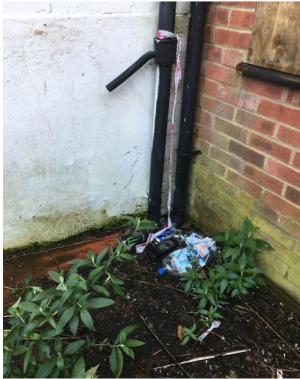
Photograph 17: Drainage infrastructure located along southern Site boundary (associated with neighbouring public house)
