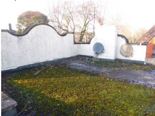
5. Astro-turf on the roof towards front of house (viewed from roof).
