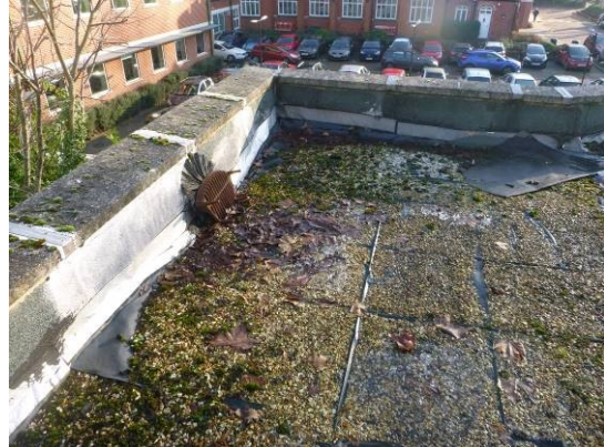
4. Gravel layer on top of bitumen flat roof around store room (viewed from roof).
