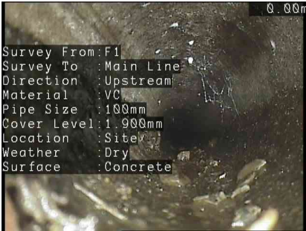
Main LineX_b1ea2241-b4df-464b-a751-1b9bd1c5c73e_20191125_145016_206.jpg, 00:00:00, 0.00 m Start node type, manhole, reference number: F1
