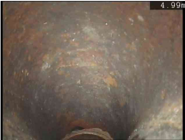
F1X_f542f806-2ee1-4d70-b3bb-59ebec874b68_20191125_175703_604.jpg, 00:01:14, 4.99 m Line deviates down
