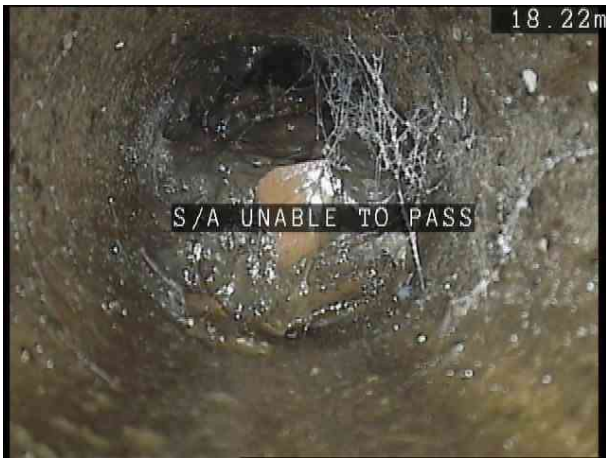
Main LineX_9175a137-e550-4076-afa4-87df49136cda_20191125_1 45719_215.jpg, 00:02:32, 18.22 m Survey abandoned, Unable to Pass
