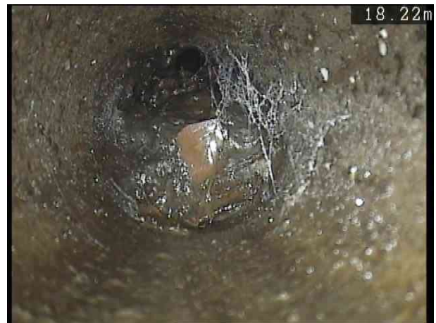
Main LineX_9a2cc2c2-2659-4514-84a9-1f36fc219581_20191125_145615_714.jpg, 00:02:26, 18.22 m Settled deposits, other, 85% cross-sectional area loss, Debris
