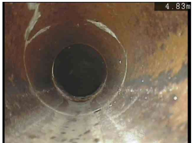
F1X_c9e00913-5fde-40ec-9ee5-e999b6c307ce_20191125_175639_021.jpg, 00:01:10, 4.83 m Fractures, multiple from 12 o'clock to 12 o'clock
