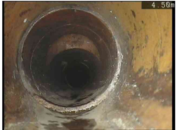
F1X_78ddbc7b-9639-4ab2-9d72-13d2d7a550ed_20191125_175454_481.jpg, 00:01:06, 4.50 m Joint displaced, medium
