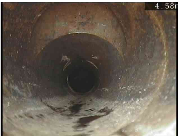
F1X_bb75f851-30d7-4288-aa69-ee090f5fe07f_20191125_17540_290.jpg, 00:01:08, 4.58 m Connection other than junction at 12 o'clock, diameter: 100mm
