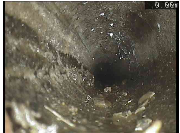
Main LineX_c6e470b9-2d3d-428f-a776-36c736051274_20191125_145234_427.jpg, 00:00:00, 0.00 m Settled deposits, coarse, 10% cross-sectional area loss
