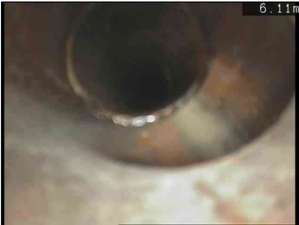
F1X_231ff565-22a5-4d0c-97a5-77decbbc0660_20191125_180143_226.jpg, 00:01:42, 6.11 m Connection other than junction at 4 o'clock, diameter: 100mm
