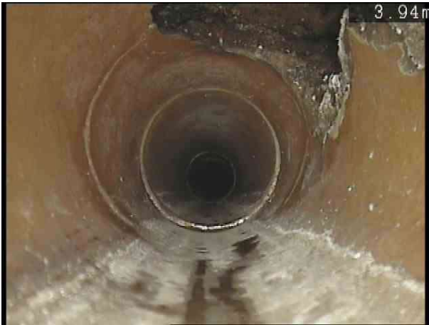
F1X_0396c4b3-f5ed-4424-a9ca-b6ae0c67a1f3_20191125_175417_276.jpg, 00:01:00, 3.94 m Fracture, circumferential from 3 o'clock to 11 o'clock
