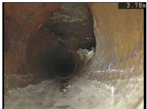
F1X_d0e06b4e-aba8-4dad-ad2e-5b22f246f8a6_20191125_175354_812.jpg, 00:00:54, 3.78 m Broken pipe from 11 o'clock to 3 o'clock, start
