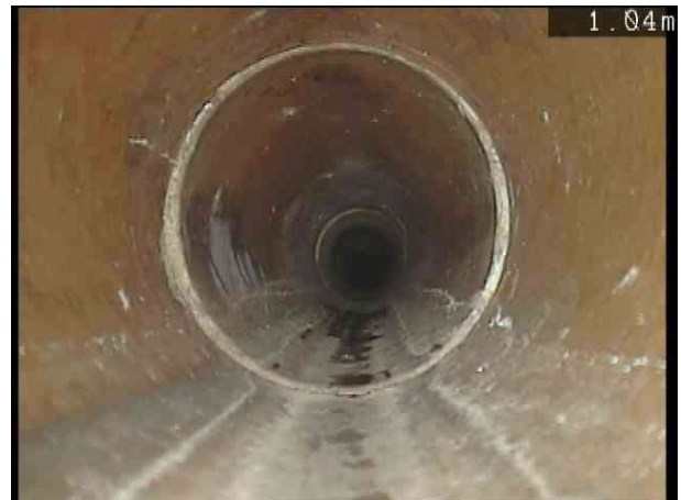
F1X_3bbeab53-0528-487b-bbd0-238e28fb5ff6_20191125_175133_215.jpg, 00:00:20, 1.04 m Fracture, circumferential at joint from 12 o'clock to 2 o'clock
