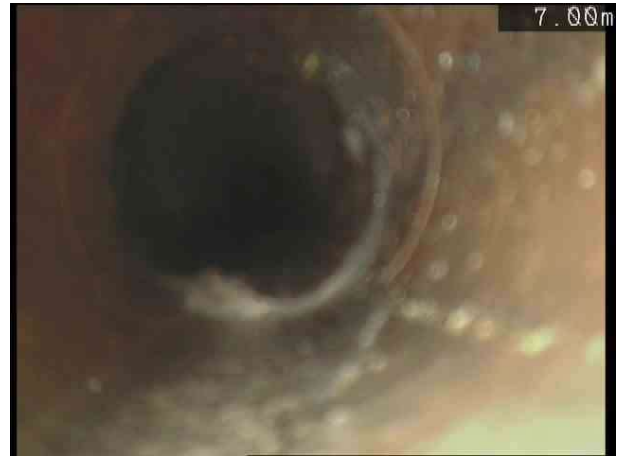
F1X_38c6b55f-6a66-4cf7-b4d5-6c4ec9efcc96_20191125_180206_623.jpg, 00:01:52, 7.00 m Fracture, circumferential at joint from 12 o'clock to 12 o'clock
