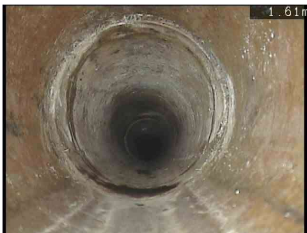
F1X_bb7ff867-2fc6-4f60-87ac-8c568a1e6035_20191125_175225_183.jpg, 00:00:27, 1.61 m Fracture, circumferential at joint from 12 o'clock to 12 o'clock
