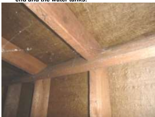
21. The largely intact paper backed felt widely cobwebbed at the ridge.
