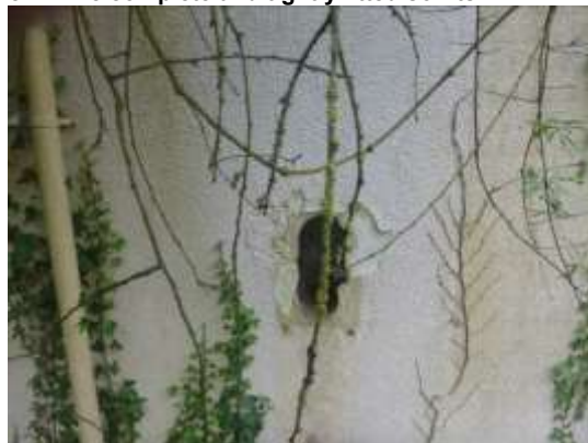
10. The hole into the wall on the front (eastern) side of the house.
