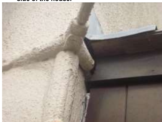
12. Cobwebbed gap at junction of the single storey extension and house.
