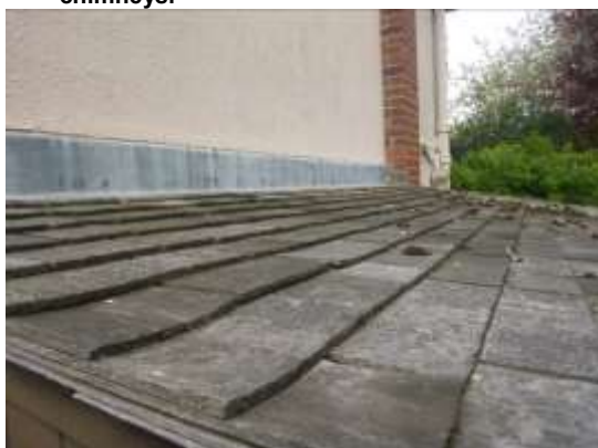
11. The timber shingles covering the single storey extension largely flat or with superficial gaps beneath.
