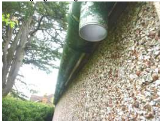
16. Slight gap beneath barge board on garage showing no signs of use by bats.
