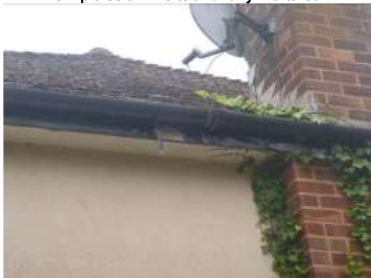
9. The flat and tight lead flashings around the chimneys.
