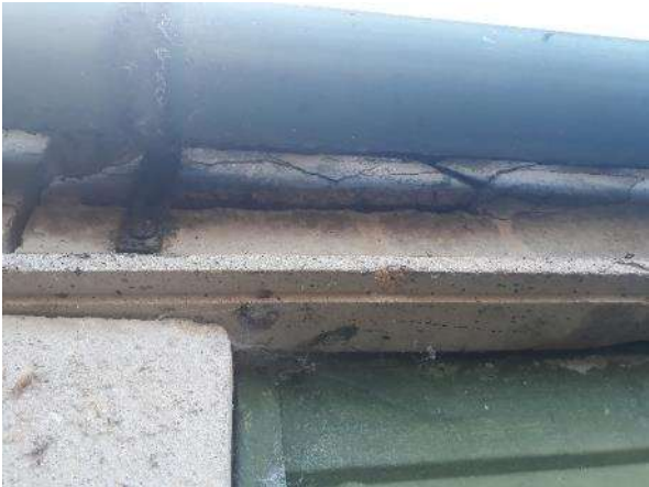
Photo 14: Cracks in concrete beam.
