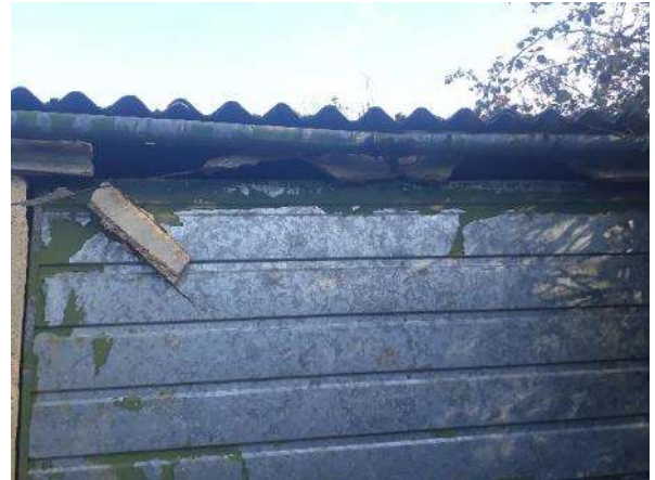
Photo 15: Broken concrete beam above garage door.
