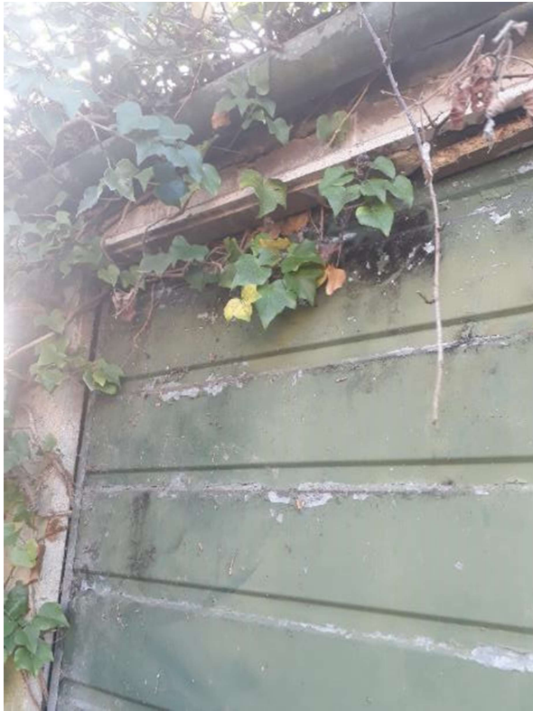
Photo 13: Cracks in concrete and ivy.
