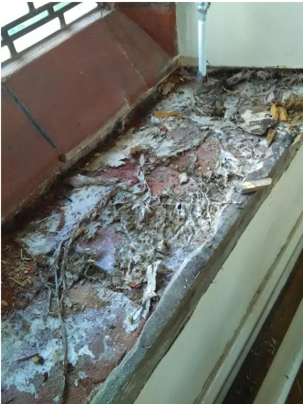
Figure 3: Exposed dry rot to window board 2.
