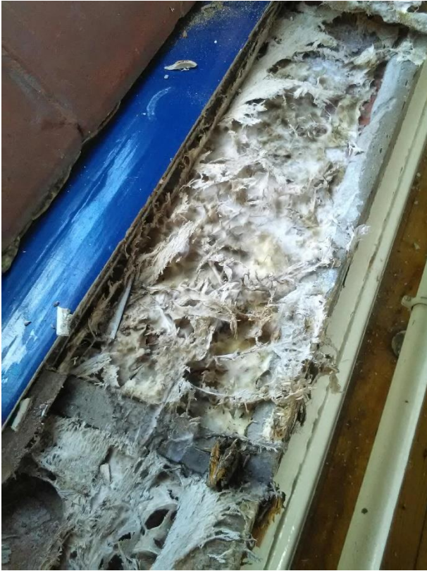
Figure 2: Exposed dry rot to window board 1.
