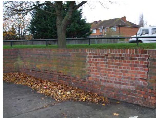
Cracking to brick retaining wall
