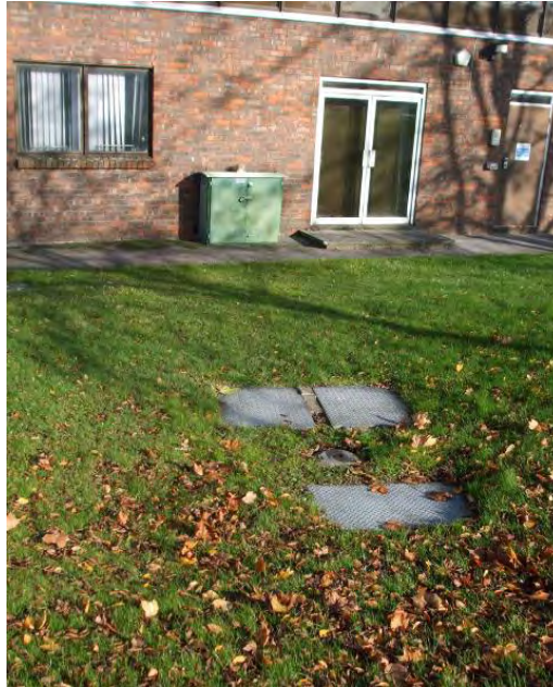
Interceptor and pump warning system..
