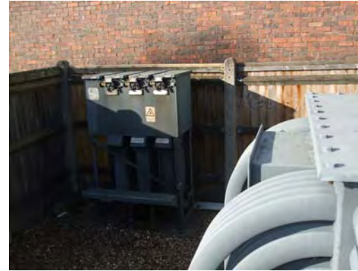
Substation oil filling point note staining on the apparatus and to the brick wall.
