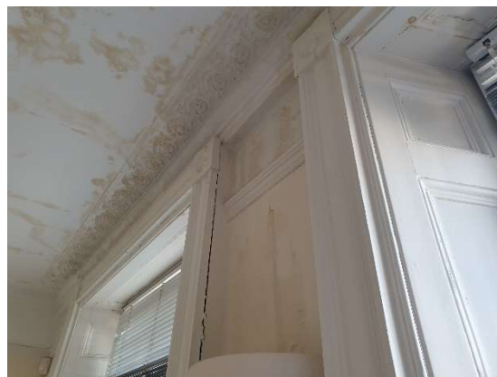
Front classroom timber window surround damage
