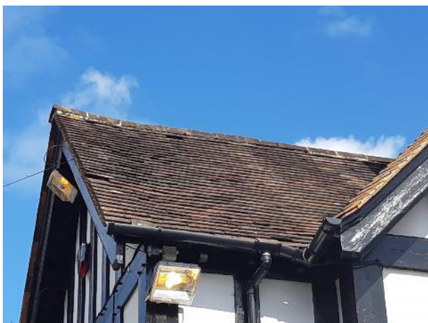
Photograph 3. Missing tiles from the south-eastern aspect of the public house's (Building A) roof.
