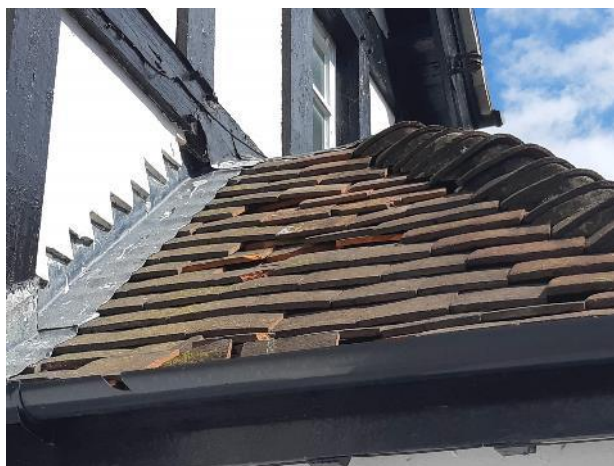
Photograph 4. Broken/missing tiles from a bay window at the south-eastern elevation of the public house (Building A).
