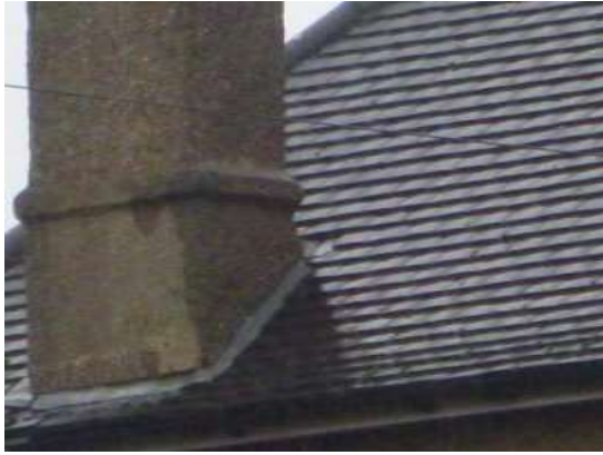
7. Gaps under roof tiles behind the chimneys.
