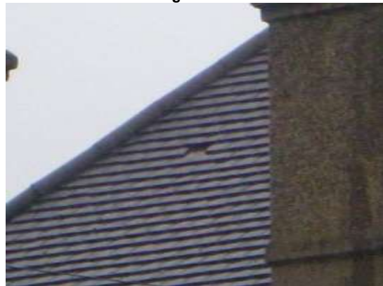
4. The one missing roof tile on the western side elevation.
