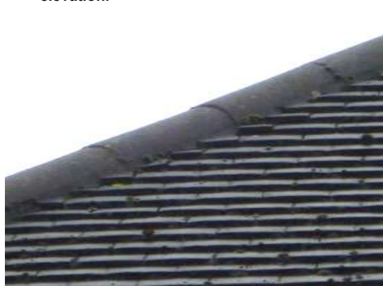
6. The superficial gaps under the tile cuts on the hip.
