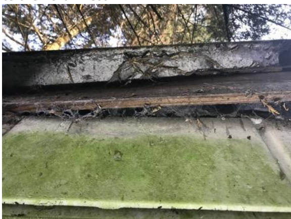
Photograph 5: Heavily cobwebbed raised fascia to the north west
