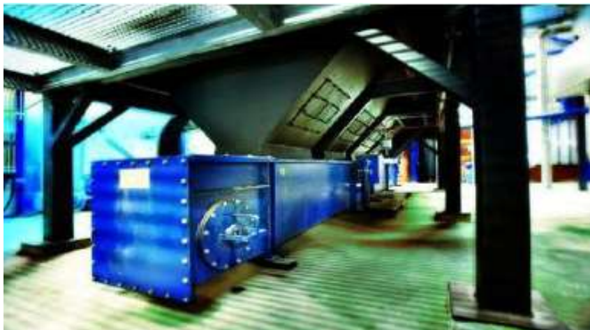
Figure 10: Wet conveyor ash
