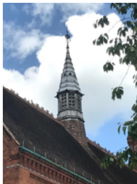
Photo 3 – Central tower with multiple lifted/missing hanging tiles
