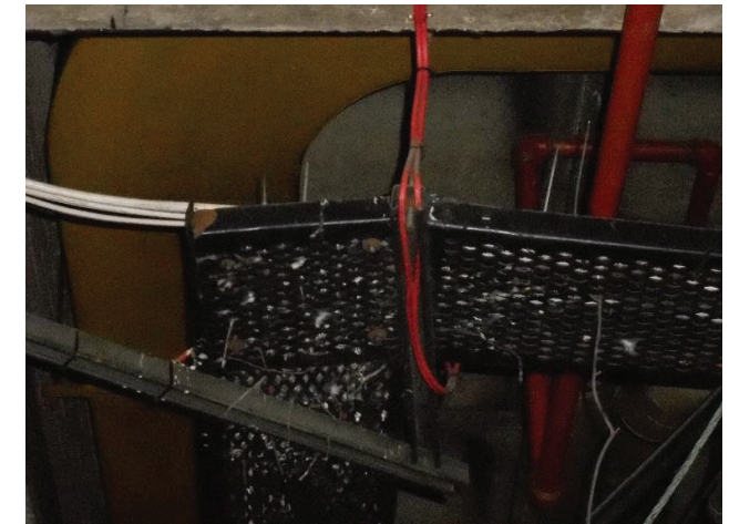
Photograph 11 Feral pigeon nesting site above metal shelf in basement area.
