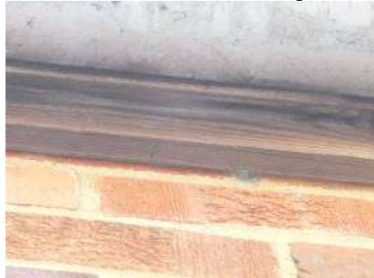
4. The narrow gap behind the barge board in places.
