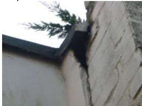
6. Large hole in the brickwork on the western side of the building.
