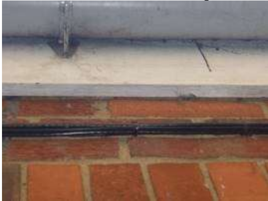
3. The tight barge boards on the northern side of the building.
