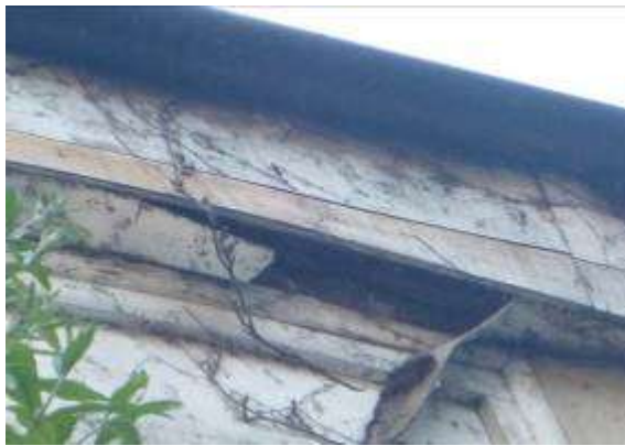
7. The rotting wooden soffit box on the southern side of the hipped roof.
