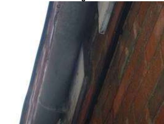
5. The missing brick above the ventilation brick but guttering in the way of easy access.
