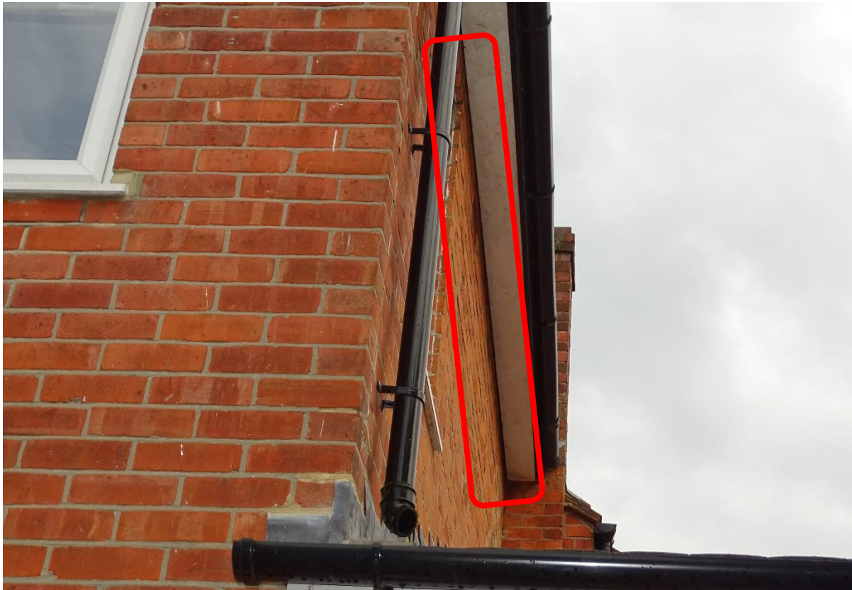
Image 3 – Eaves coverings across the West facing elevation which offers suitable access features of value to bats which would lead into the enclosed void section of the eaves which would be a suitable seasonal daytime roosting environment
