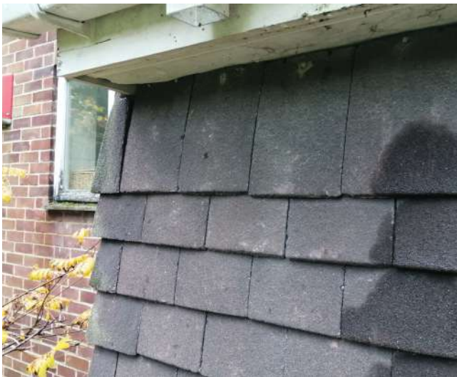
Image 15: Gap beneath corner hanging tiles
