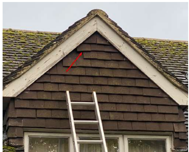
Image 4: Location of missing tile gap inspected by endoscope
