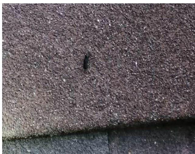
Image 17: Droppings found stuck to hanging tiles
