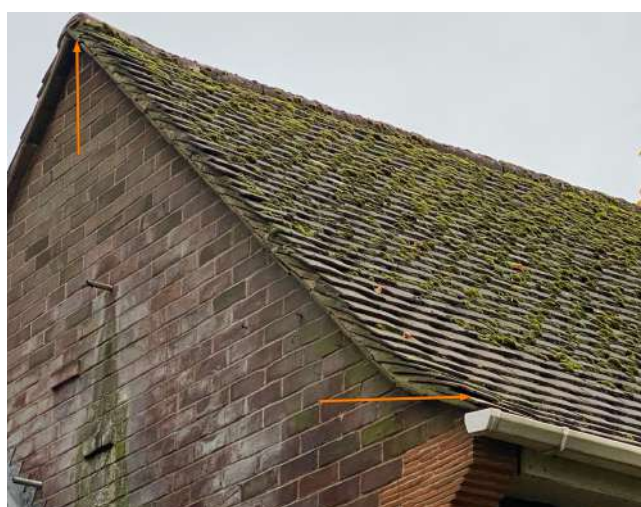
Image 5: Lifted verge tiles and mortar gap on the eastern elevation
