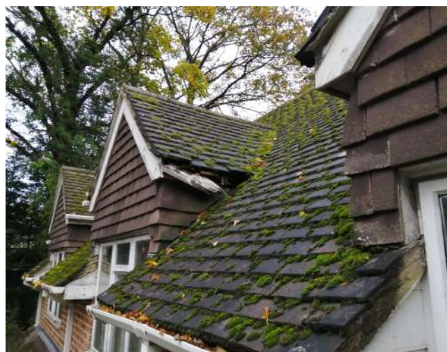
Image 11: Coverage of moss on roof tiles
