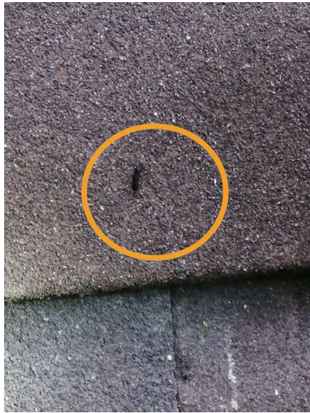
Droppings found stuck to hanging tile on the eastern elevation:
