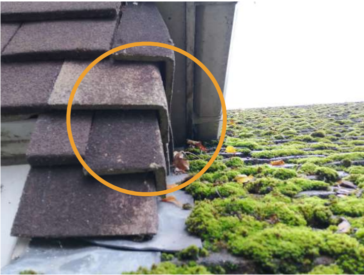
Droppings found under hanging tiles on the western elevation:
