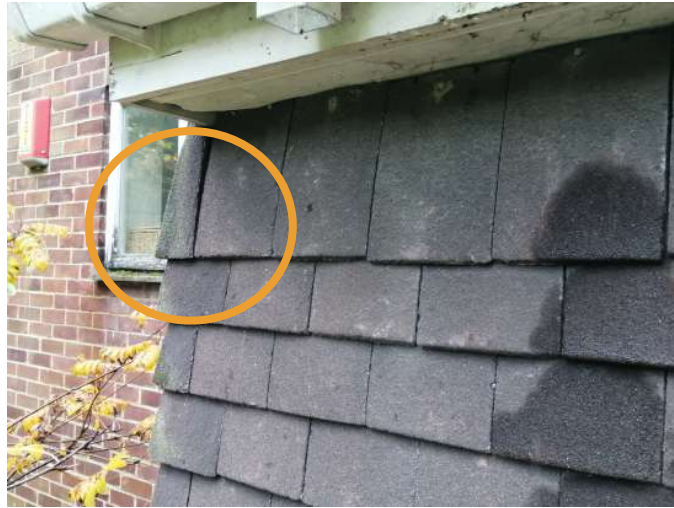
Droppings found under hanging corner tile on the eastern elevation:
