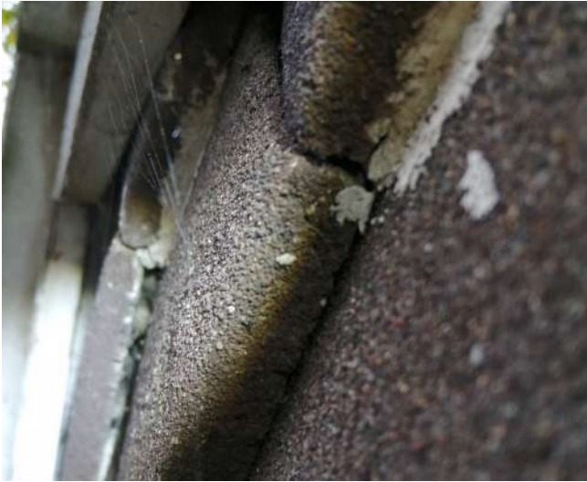
Image 7 : Light coverage of cobwebs over gap beneath hanging tiles
