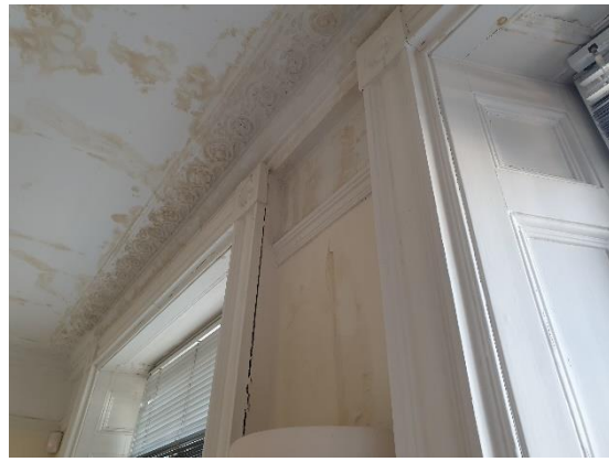
Front classroom timber window surround damage
