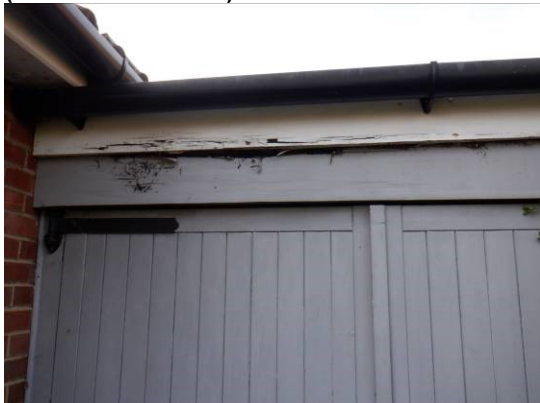
15. Weathered timbers on front of garage (front elevation).
