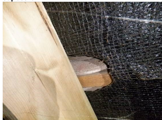
18. Small hole in bitumen roof lining.
