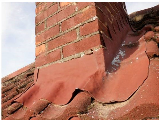
7. Slightly raised lead flashing around chimney (southern elevation).
