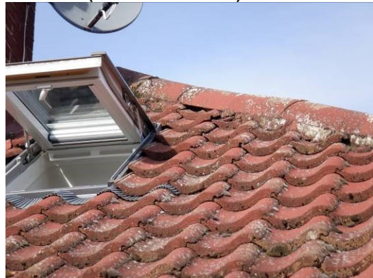
6. Missing piece of hip mortar (southern elevation).
