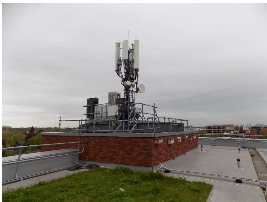
Figure 2. Photograph of existing mast (to be retained) & communications apparatus
