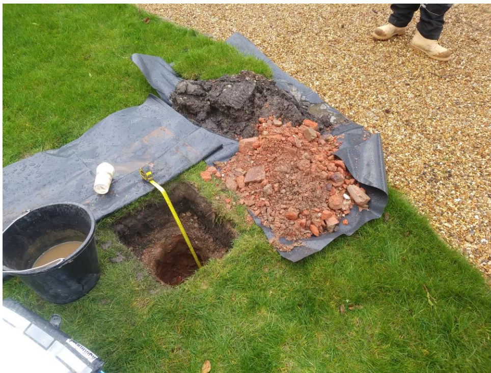
Photo 24: TP104 – membrane at 0.70m (not visible due to water ingress)
