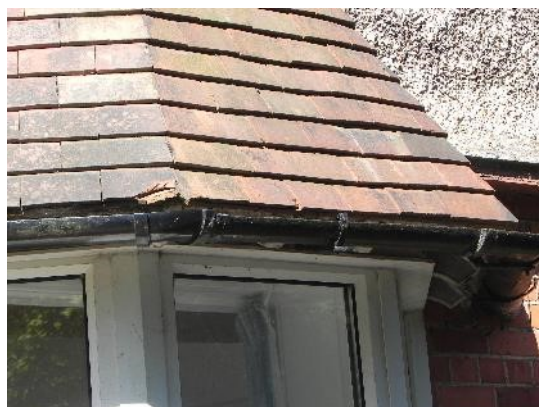
40. Tile cracked to edge of bay window roof.
