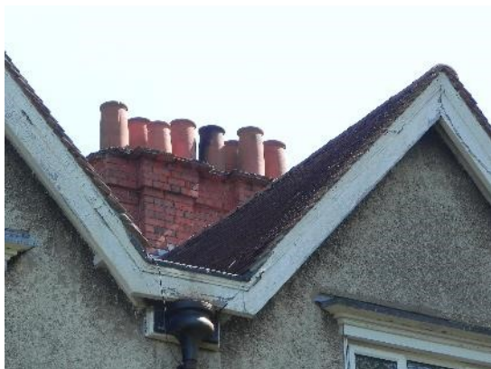
33. Mortar between chimney bricks missing in places (western elevation view).
