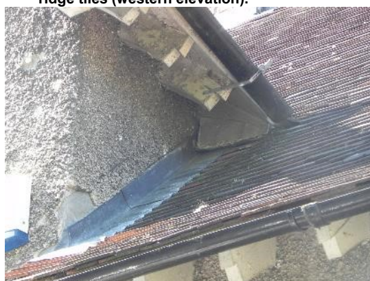
22. Lifted tiles at end near gable (eastern elevation).
