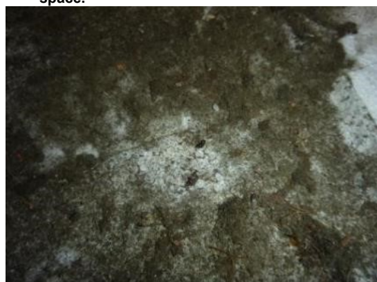
64. Further medium-sized bat droppings on floor of roof space.
