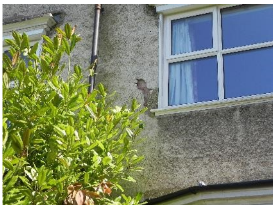
17. Large area of pebbledash cracking near second-story window (western elevation).
