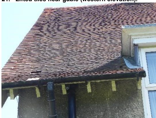
23. Missing tiles (western elevation).
