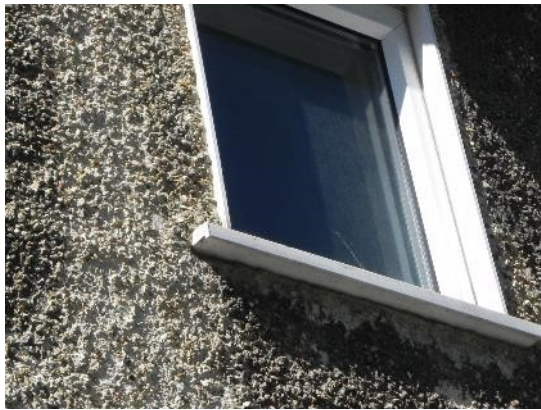
9. Gap between windowsill and pebbledash to second-storey window (eastern elevation).
