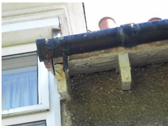
31. Slight gaps between soffits and pebbledash render (southern gable end).
