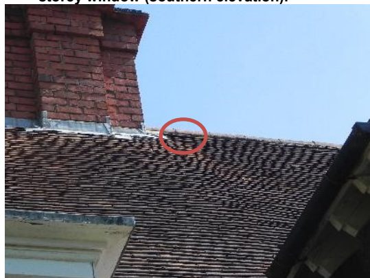
20. Further missing tiles near left chimney and ridge tiles (western elevation).
