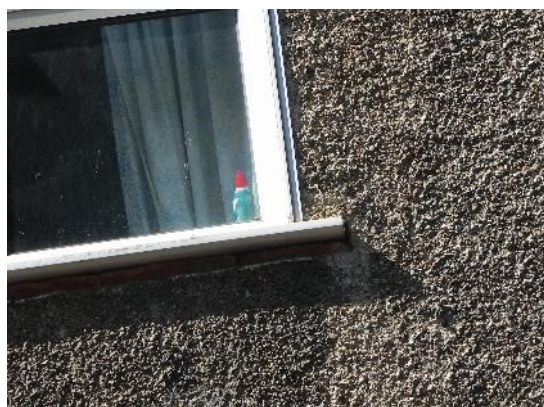
8. Gaps between second-storey windowsill, brickwork and mortar and pebbledash (eastern elevation).
