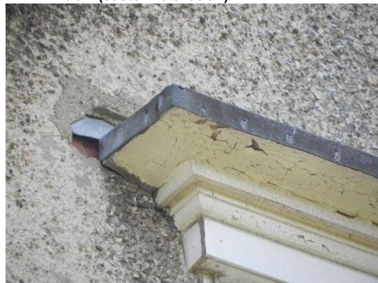
12. Crack in pebbledash creating gap between wall and gable window felt (western elevation).
