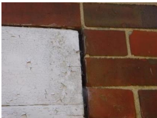
49. Gap between timber and brick to garage front (eastern elevation).
