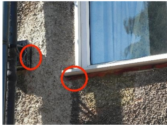
10. Gaps between downpipe fixture and windowsill and brickwork beneath to second-storey window (eastern elevation).
