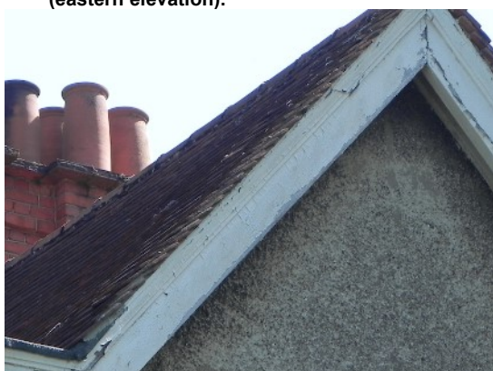
37. Lifted tiles (western elevation).
