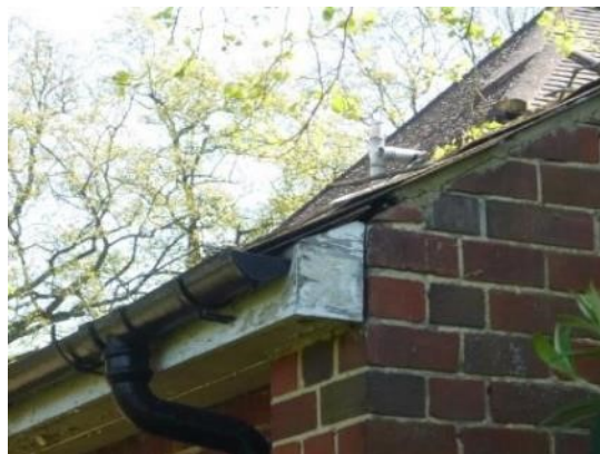
48. Gap in missing mortar to garage where brick wall meets roof (western elevation).
