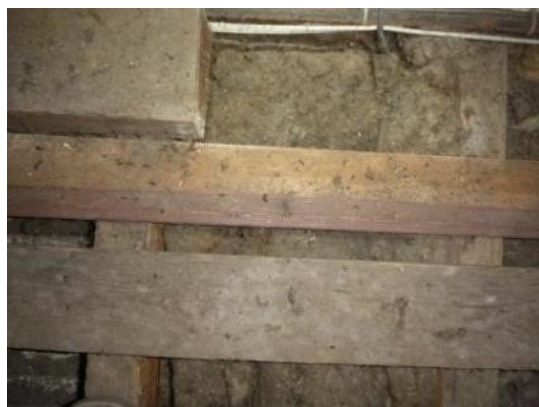
66. Further medium-sized bat droppings on floor of roof space.
