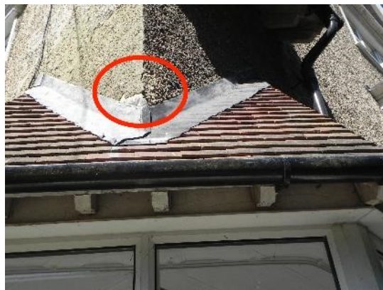
42. Crack in wall above bay window roof.
