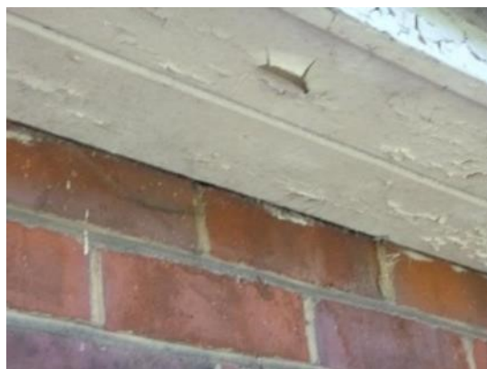
50. Narrow gap between the soffit and the wall (northern elevation).
