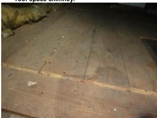
63. Further medium-sized bat droppings on floor of roof space.
