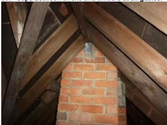
61. Gaps between bricks and timbers to internal roof space chimney.
