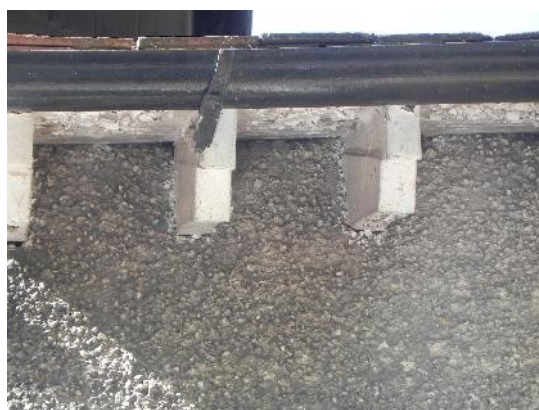
30. Slight gaps between soffits and pebbledash (northern gable end).
