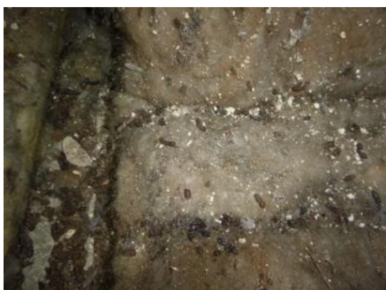
69. Concentration of 50-100 large bat droppings on roof space flooring.
