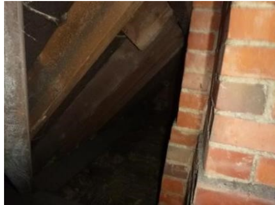
60. Narrow gaps either side of chimney/water tank.
