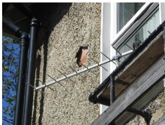
18. Large area of pebbledash cracking near second-storey window (southern elevation).
