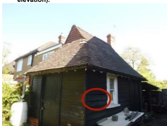
54. Loose feather boards to shed (south-western elevation).
