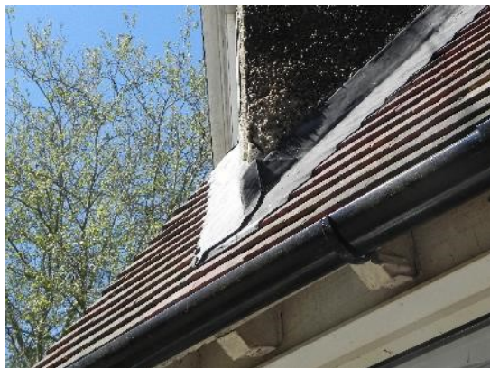
41. Potential access through loose flashing if tiles beneath present gaps.
