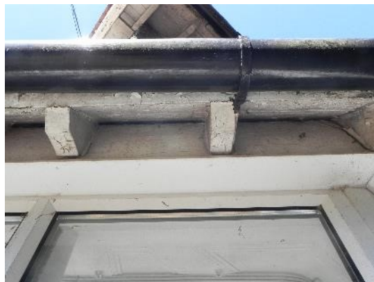
44. Further gap between eaves and bay window.
