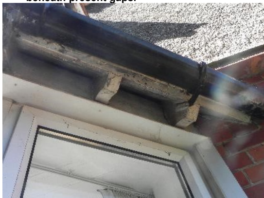
43. Gap between eaves and bay window.
