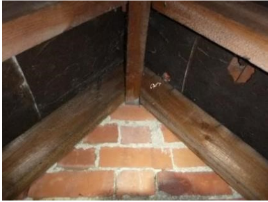
57. Internal roof space - signs of damp and cobwebs to ridge.
