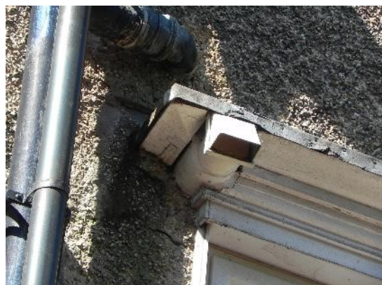
16. Gaps between flue, felt and roof to second-storey window (eastern elevation).
