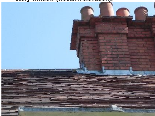
19. Lifted and missing tiles near left chimney (western elevation).
