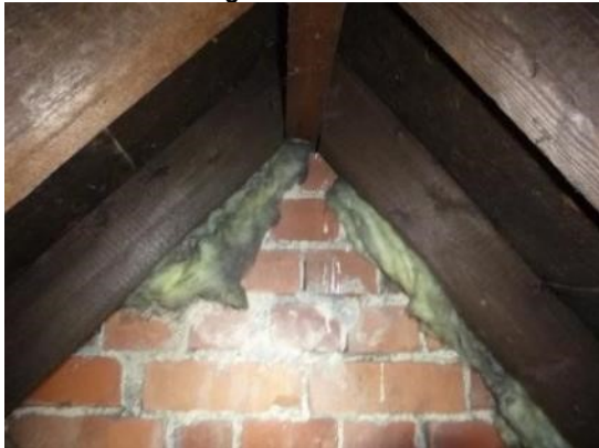
59. Gaps between bricks and timbers at all gables.
