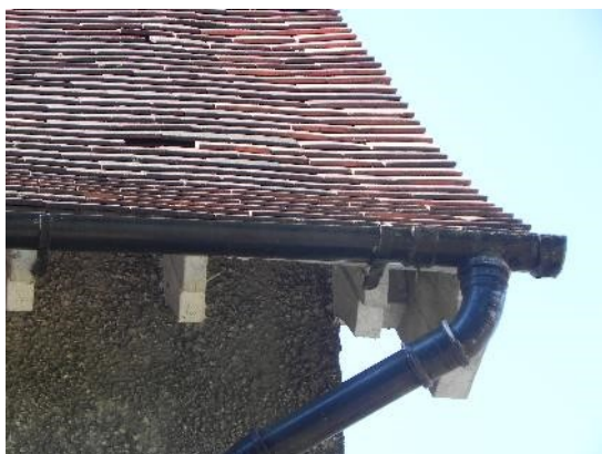
25. Missing and lifted tiles (eastern elevation).
