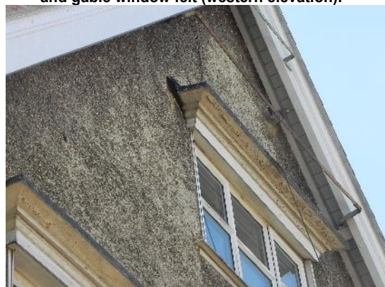
14. Large gap between gable window felt and wall (northern elevation).
