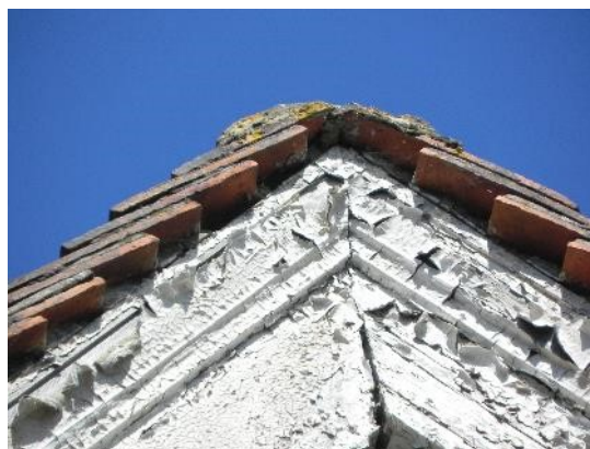
26. Gaps at and around gable apex where mortar between tiles has crumbled (southern elevation).
