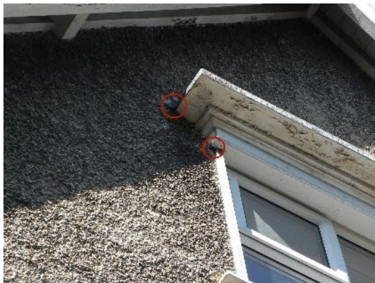
11. Gap to window edge and where flashing is loose (eastern elevation).
