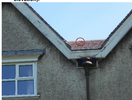
28. Cracked ridge tile from western view.
