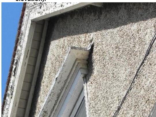
15. Gap between gable window felt and wall (eastern elevation).
