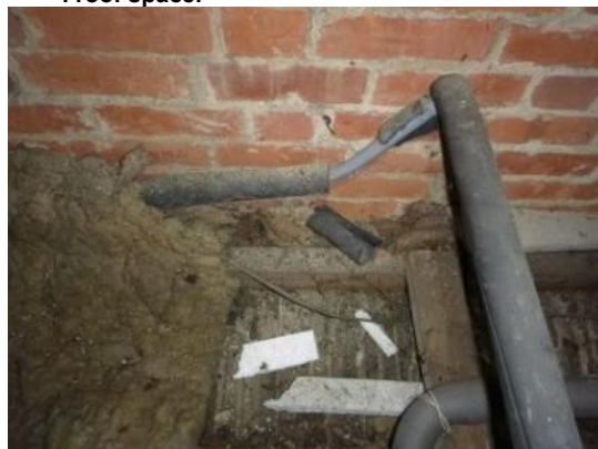
68. Further medium-sized bat droppings hanging from wall of roof space.
