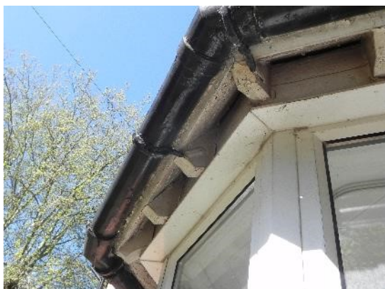
45. Further gap between eaves and bay window.
