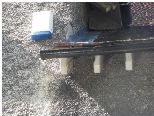
36. Gap between lifted gable soffit and tiles/ flashing (eastern elevation).
