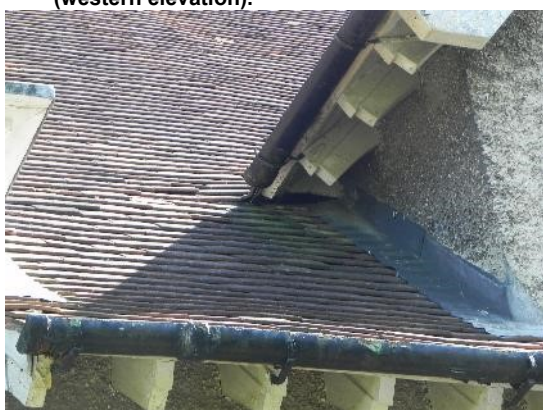
21. Lifted tiles near gable (western elevation).
