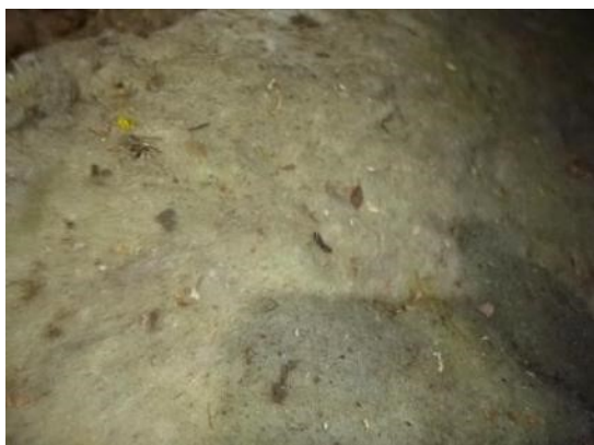
65. Further medium-sized bat droppings on floor of roof space.
