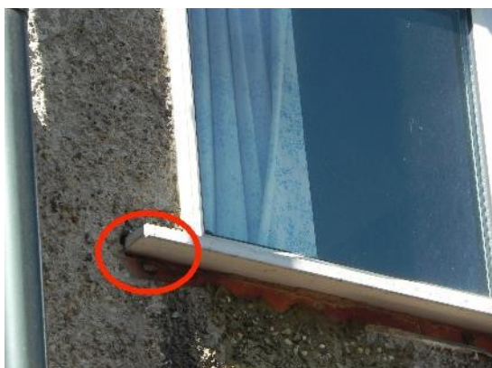
7. Gaps below and around windowsill on second-storey window (eastern elevation).
