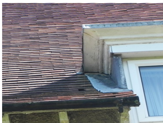
38. Felt starting to lift on dormer roof edges and soffit not flush with flashing.
