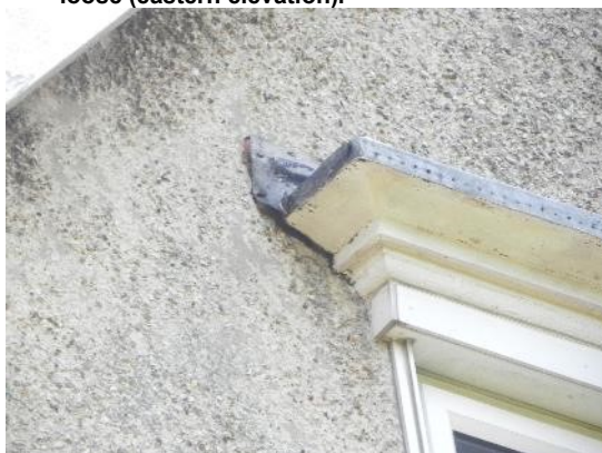
13. Further gap and cracked pebbledash area where felt for gable window meets wall (eastern elevation).
