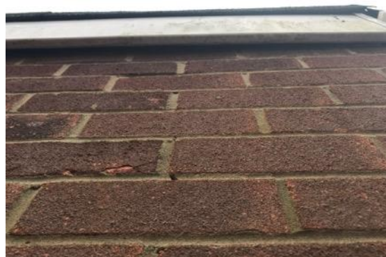
Photo 4: Gap under fascia board on single storey extension to the north
