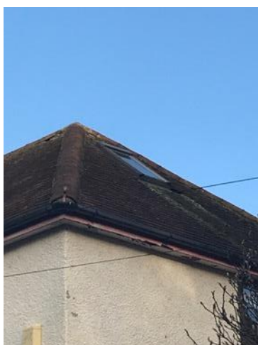
Photo 5: Missing mortar under ridge tiles and lifted tiles around roof window
