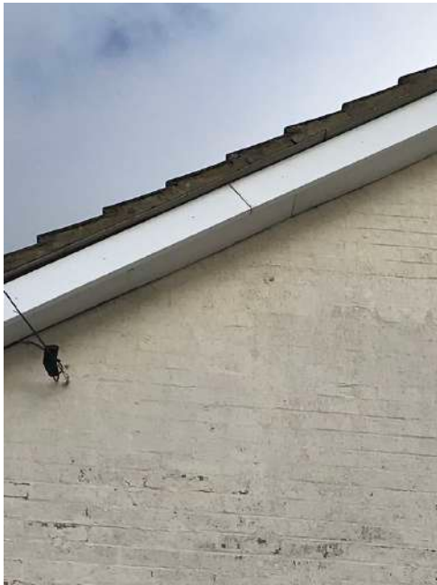
Plate 6: Gap Between Soffit and Wall South Face
