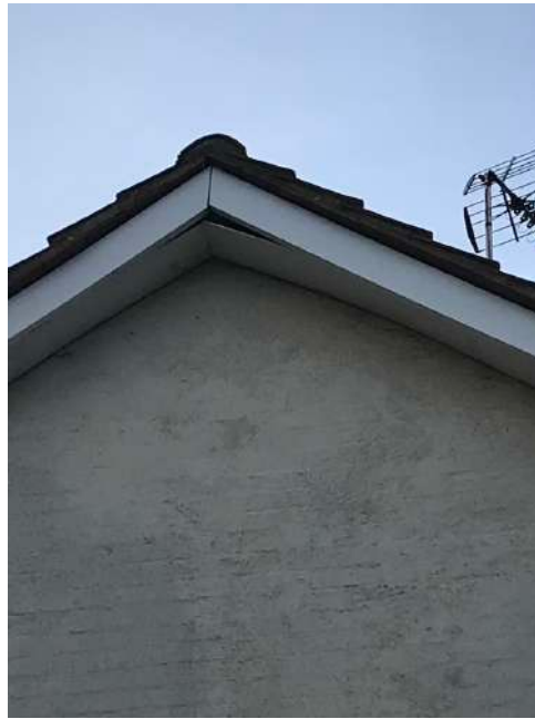
Plate 7: Gap in Soffit Board North Face
