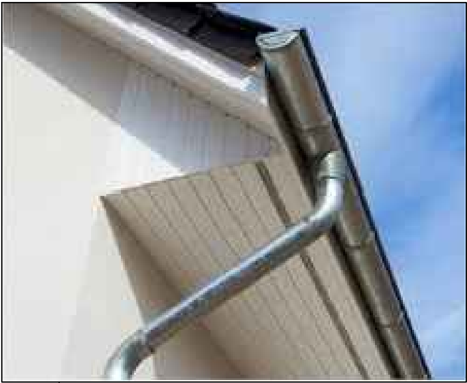
Galvanised gutters and downpipes
