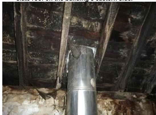
12. Daylight around a flue pipe close to eaves in the slate roof on the eastern side of the building.
