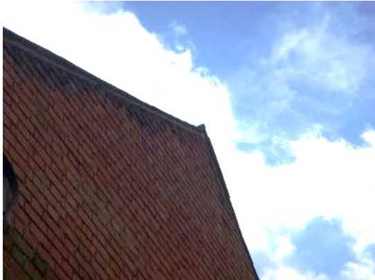
3. The intact mortar at the northern gable of the slate roofed part of the building fronting St John's Street.
