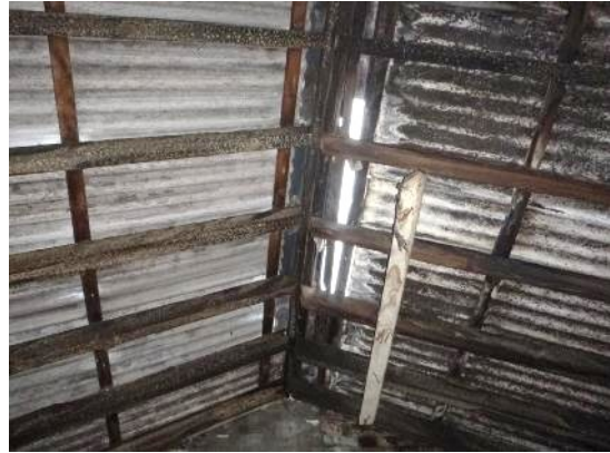
8. Gaps in the corrugated sheeting at the ridge.
