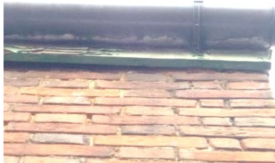
6. Gaps between the barge board and brickwork on the front (eastern) elevation of the slate roofed part of the building fronting St John's Street.
