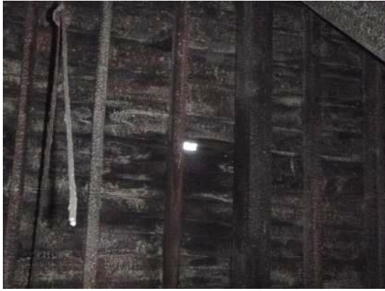
13. Daylight visible through the sarking boards in the slate roof on the eastern side of the building.
