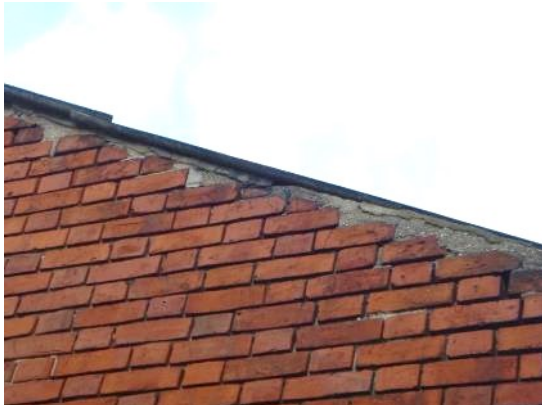
5. Gaps in the mortar between the sheet roof and brickwork.
