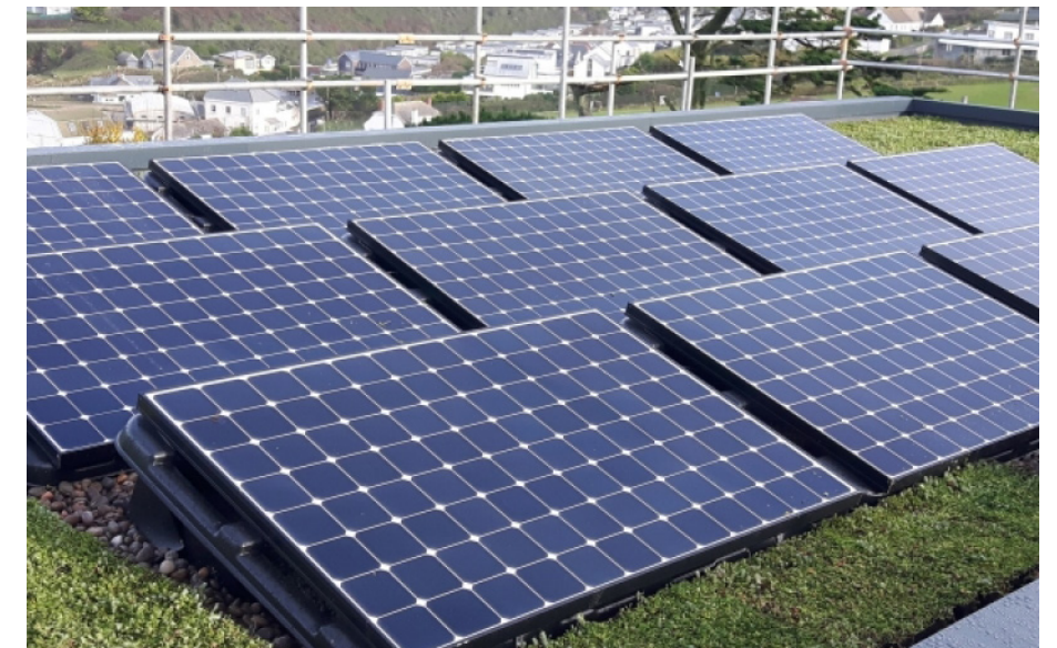
Rooftop PV panels
