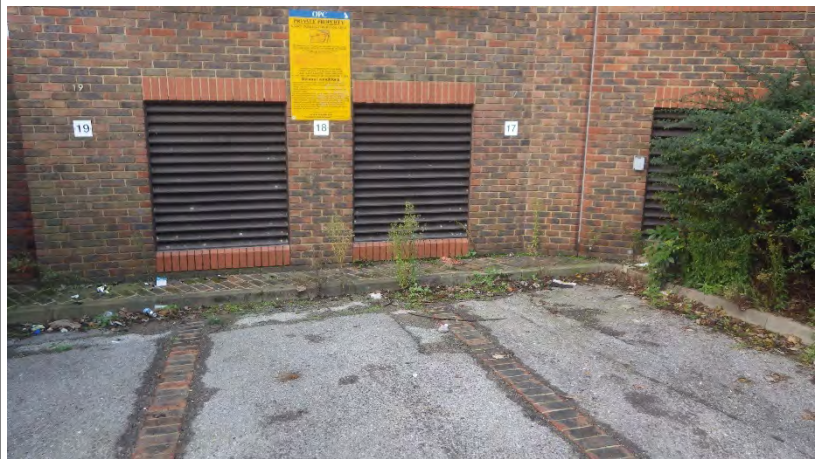
Photograph 6: Some ephemeral vegetation growing out of the concrete with the basement level in the rear of the photograph. This grille is covered in a mesh preventing access to bats and birds.
