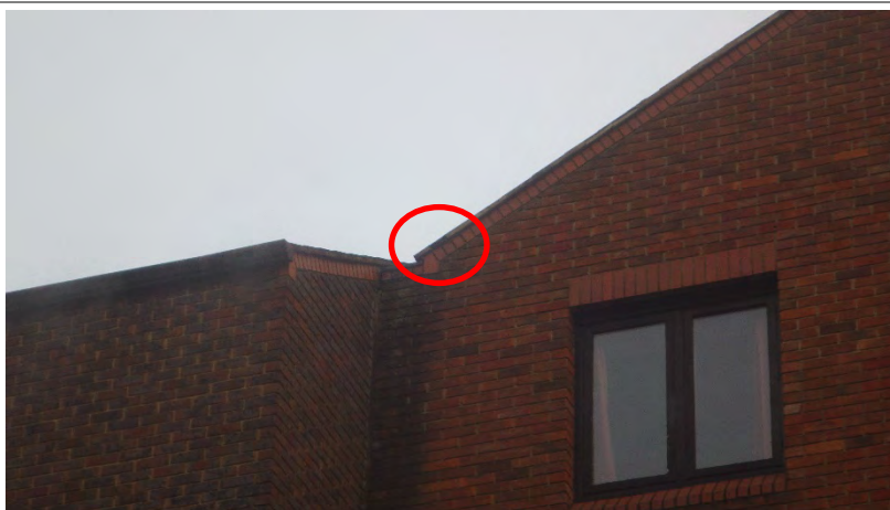
Photograph 8: A potential roosting feature (TN4) on the western gable of building B1.
