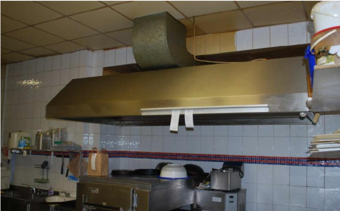
Figure 2 – The Kitchen Extraction and Internal Ductwork in the Pizzeria at 40 Oxford Road
