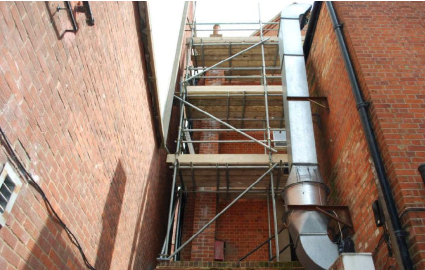
Figure 3 – The External Ductwork on the North Elevation of 40 Oxford Road
