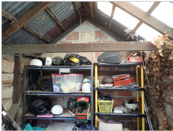
Photo 19 Internals of Building B2
