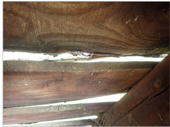
Photo 20 Large gaps showing daylight to Building B2
