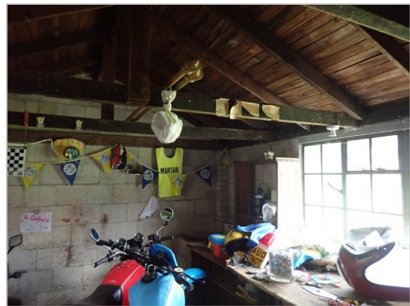
Photo 22 Internals of Building B3
