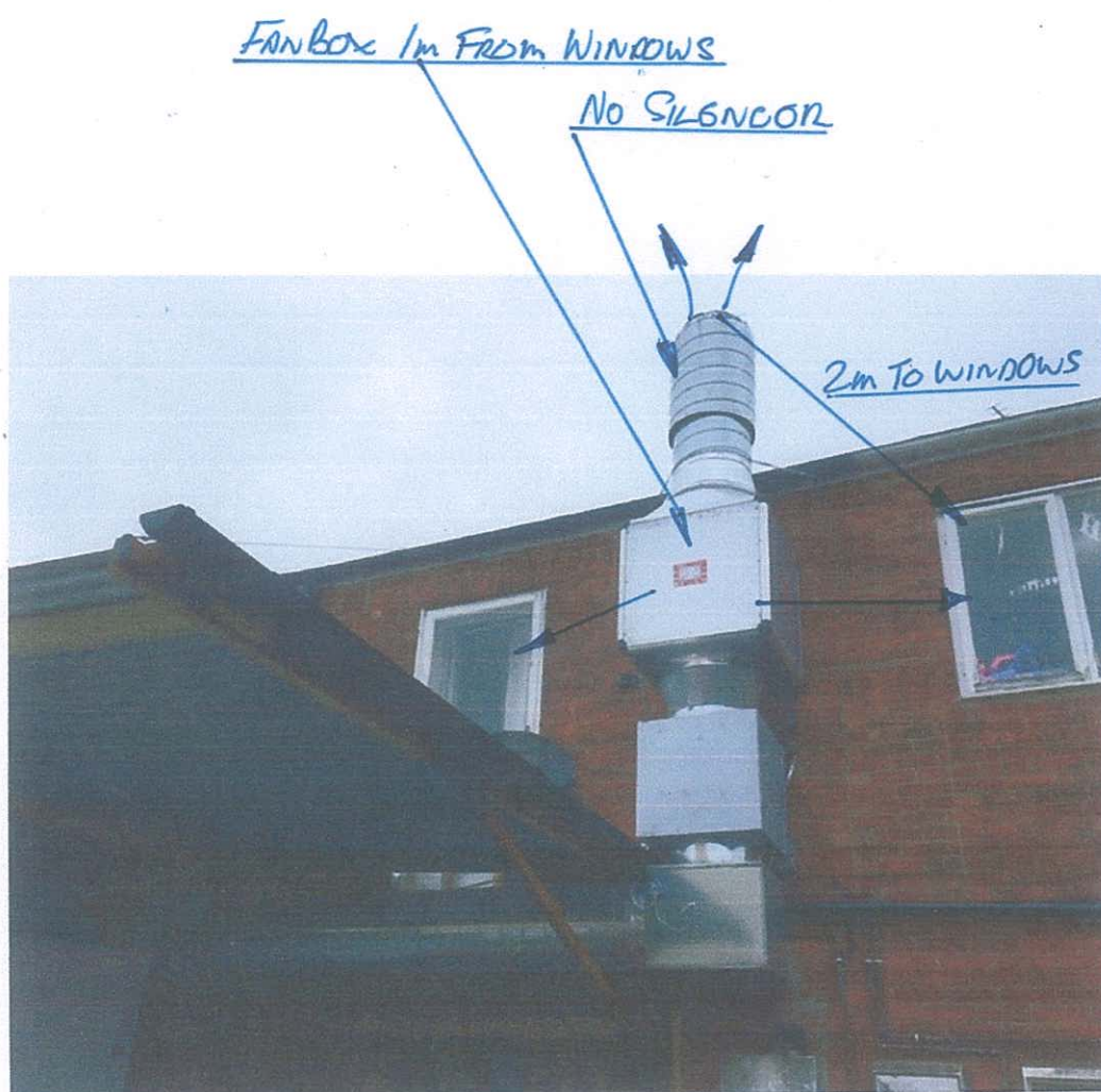
EXISTING EXTRACT VENTILATION System
