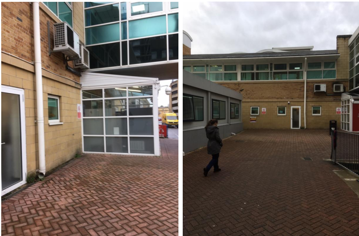
Fig.4: Photos demonstrate locations of existing external condensers.
