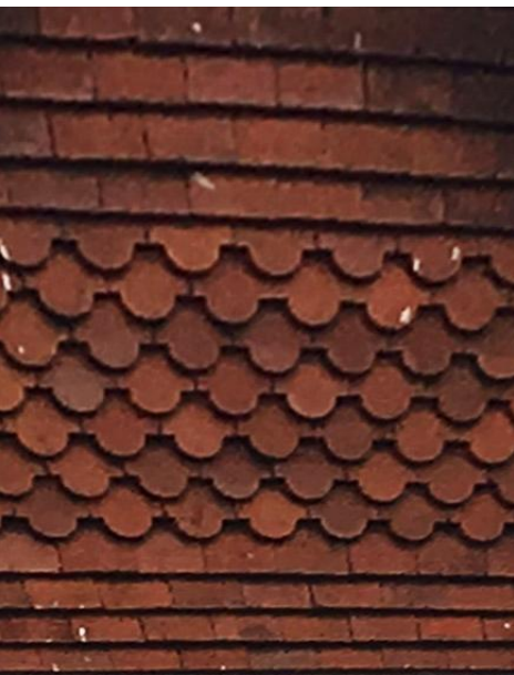
EXISTING TILE PATTERN
