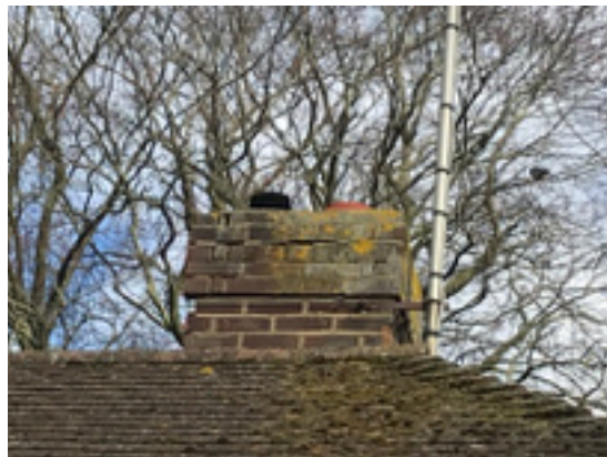
Photo 4: Gaps in brickwork on chimney
