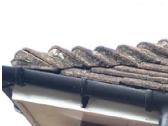
Photo 5: Gaps around hip tiles
