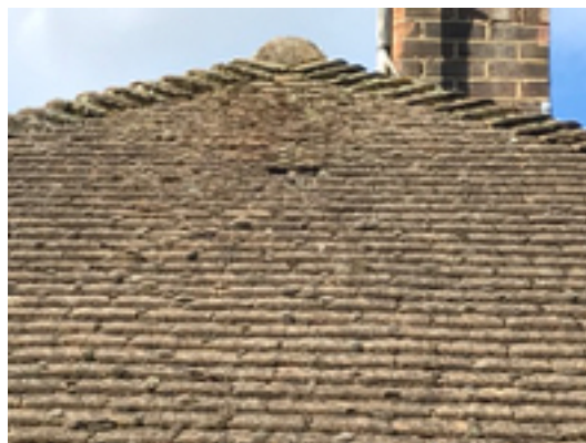
Photo 6: Missing tile on southern elevation
