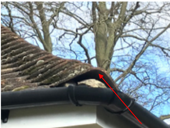
Photo 3: Missing mortar from hip tile
