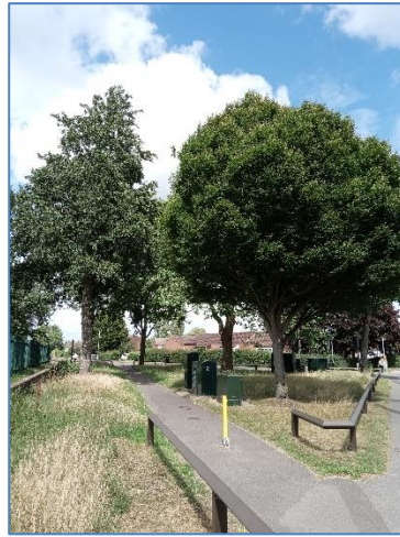
Fig 8. Existing cabinets next to proposed equipment location.
