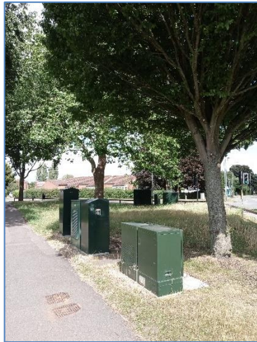
Fig 7. Existing cabinets next to proposed equipment location.
