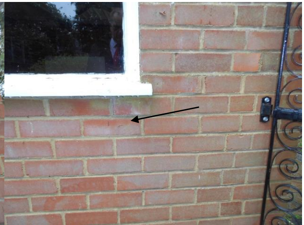
Detached garage- Stepped tapered cracking of up to 1mm was noted to the brickwork bottom right of the left hand front window.
