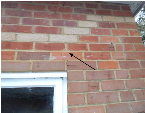
Detached garage- Stepped tapered cracking of up to 1mm was noted to the brickwork top right of the left hand front window.
