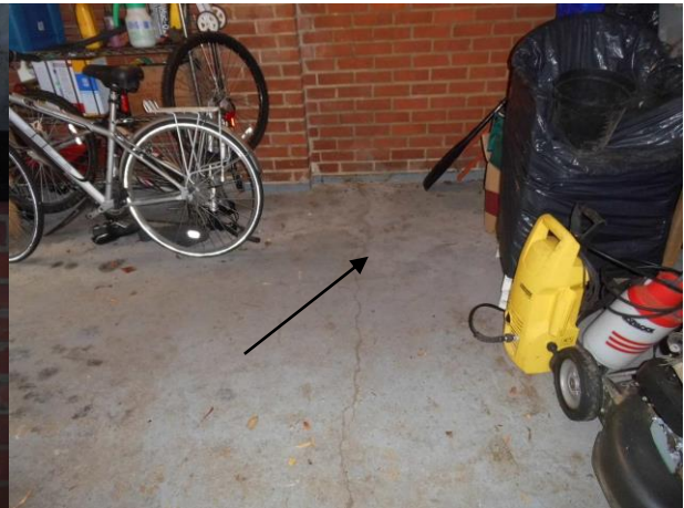
Detached garage- Front to rear to the centre of the garage is a crack to the concrete floor, with signs of a slope to the rear right corner, with maximum crack widths of 2mm.
