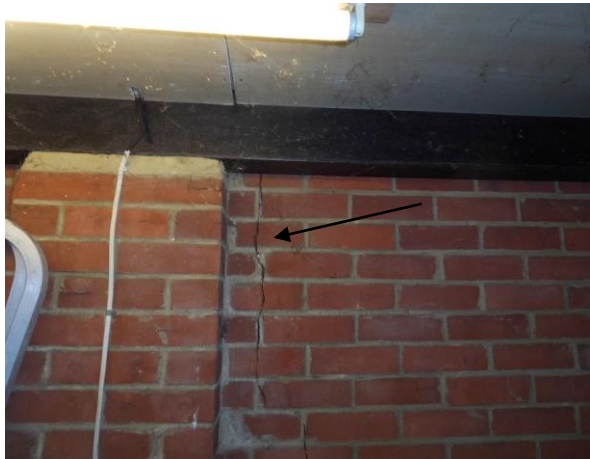
Detached garage- Vertical and stepped tapered cracking of up to 7mm was noted to the brickwork rear centre elevation of the garage.
