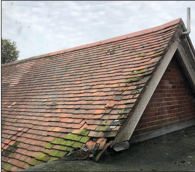
Figure 5: Missing and slipped tiles on Void D.
