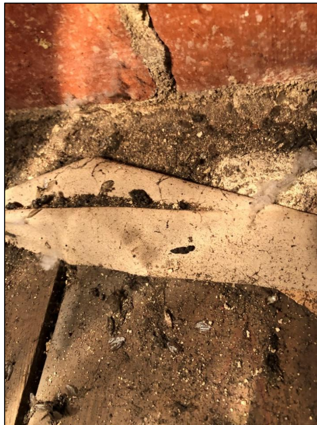
Figure 10: Bat dropping found under ridge in Void A
