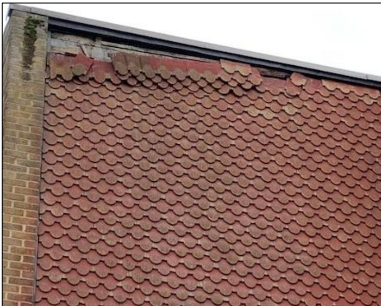
Figure 6: Slumped and broken hanging tiles on east elevation.
