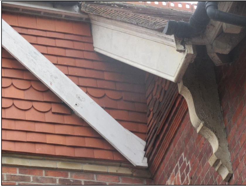
Figure 7: Gaps underneath tiles on north and west elevations.
