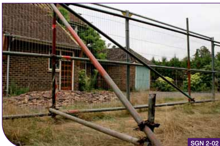
Heras fencing wired to scaffold braced posts is a robust and effective interpretation of the BS specification.
