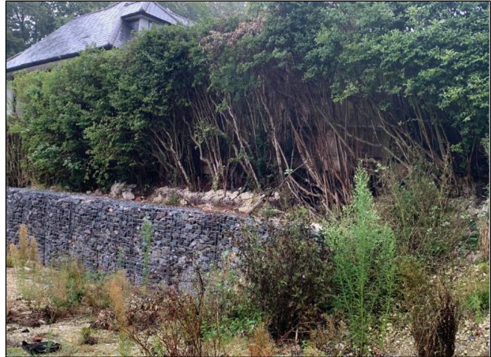
Figure 6 – Existing damaged hedging on northern boundary
