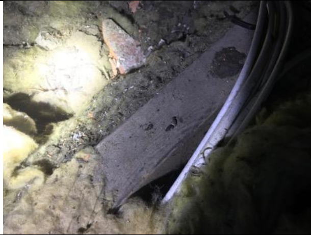
Photo 13: 3 very old bat droppings in loft
