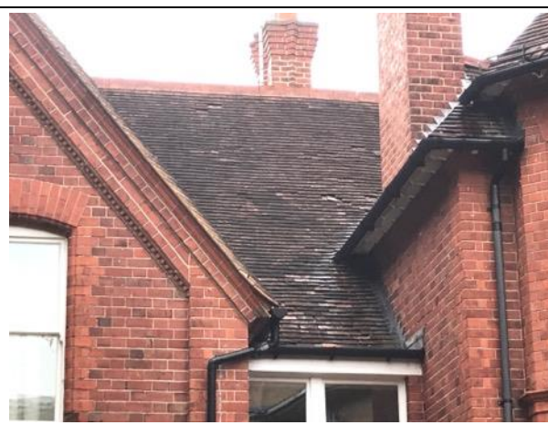
Photo 10: Many broken/ slipped tiles
