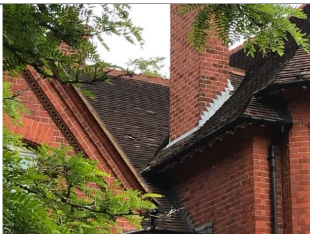
Photo 16 - Missing tiles on central section of southern elevation
