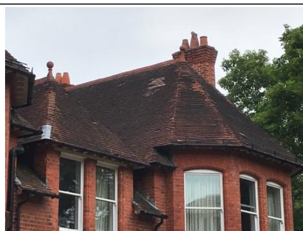
Photo 17 – Missing tiles on east section of southern elevation
