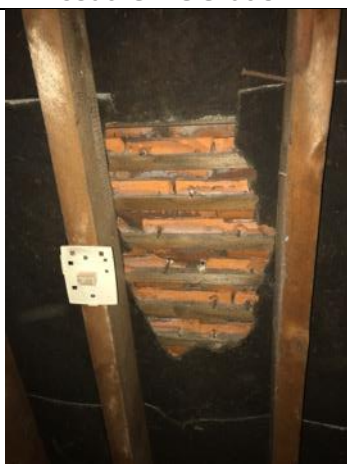
Photo 18: Hole in felt within loft exposing tiles
