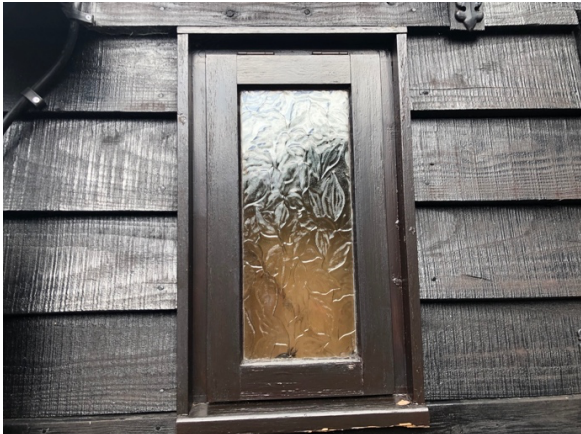
Photo 4 – Cloakroom window to be replaced
