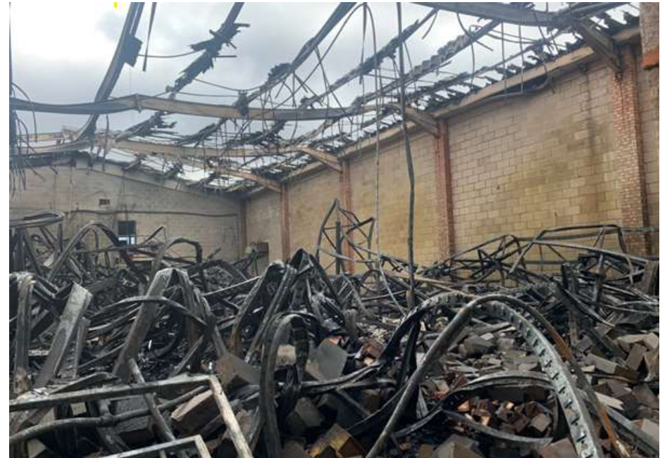
FIGURE 1 FIRE DAMAGE WITHIN UNIT 1
