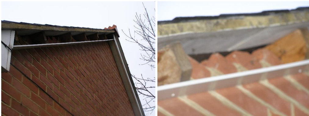
missing board on south elevation of dwelling 3 with recess space
