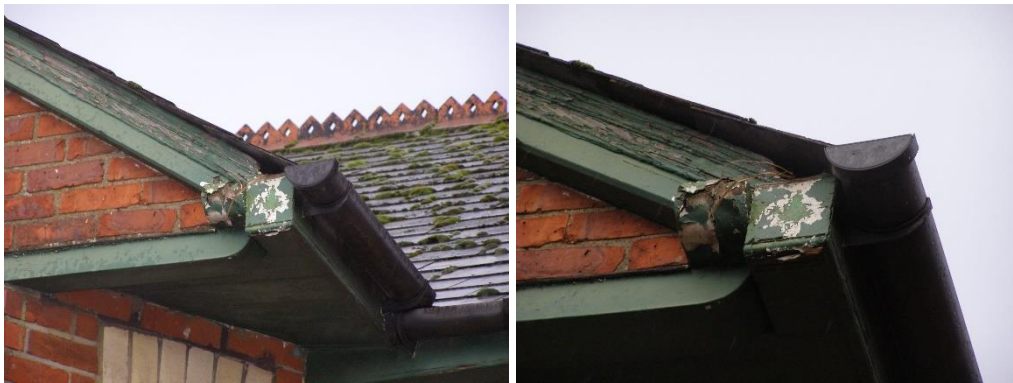
worn/weathered board with nesting material noted on western elevation of dwelling 1
