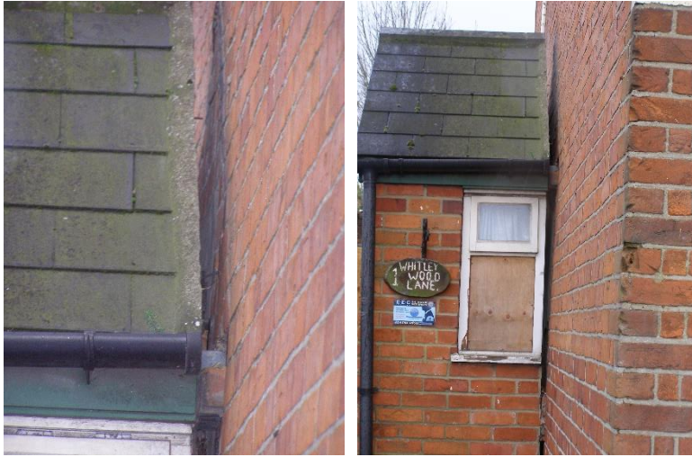
porch coming away from dwelling wall no 1
