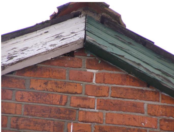
hole in upper gable wall of eastern elevation
