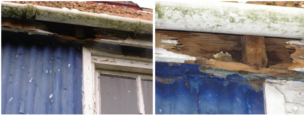
hole and weathered soffit at rear of play barn
