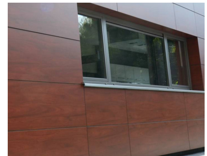
Fig. 4.22.3 - Rainscreen Panels With Fake Patterns Are Not Acceptable
