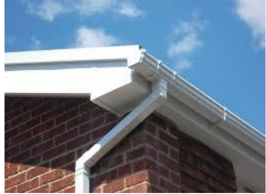
WHITE PVC GUTTERING AND DOWN PIPE
