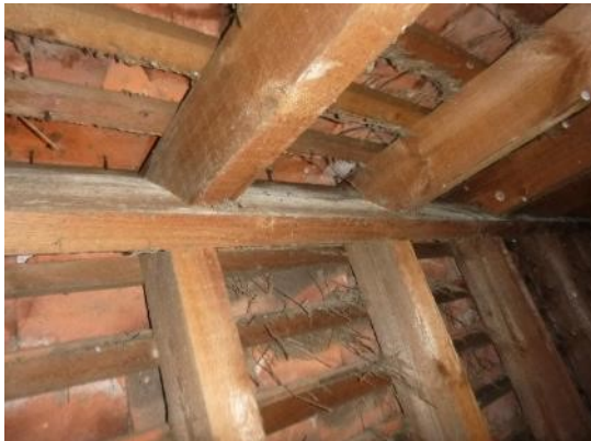
13. Unlined roof, with underside of roof tiles exposed; remnants of old straw insulation.
