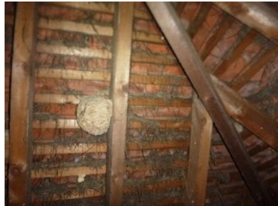
20. Old wasp nest present in the roof void.
