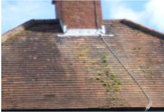
9. Slightly lifted tile below the ridge next to the chimney; intact hip tiles and mostly flat roof tiles.
