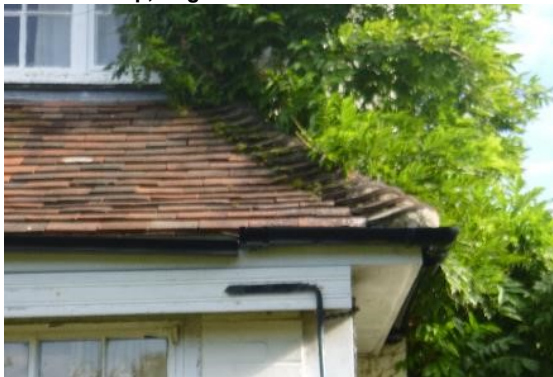
7. Uneven roof tiles on top of hipped roof to the rear of the house; gaps in mortar under the hip tiles.
