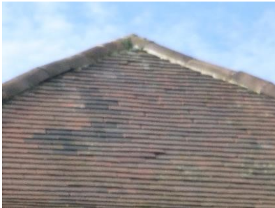
3. Uneven roof tiles to the front of the house.
