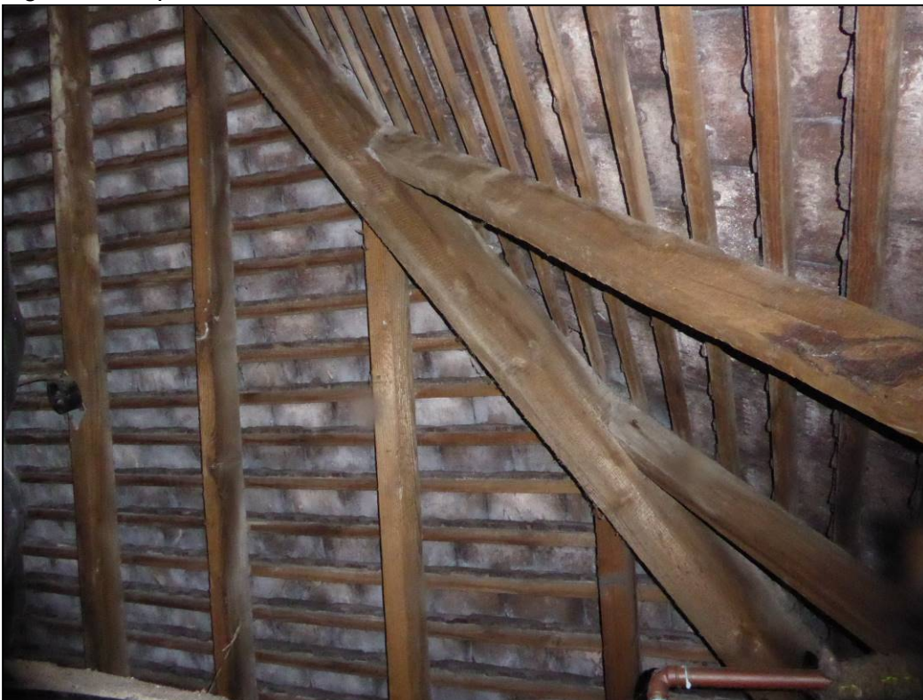
Figure 16. Exposed roof tiles. 34 Mill Road, Caversham. 19.08.20
